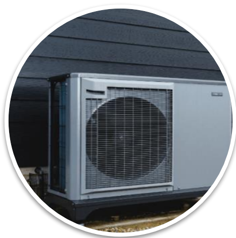
Electric heat pump
